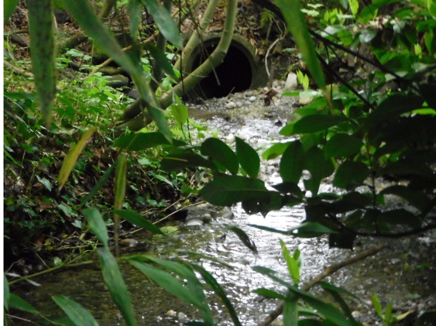
Image 7: Downstream flows are conveyed through this well-defined and protected open channel
