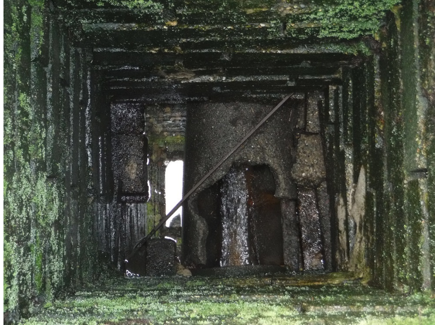
Image 5: Concrete pipe conveys flows through this CB
